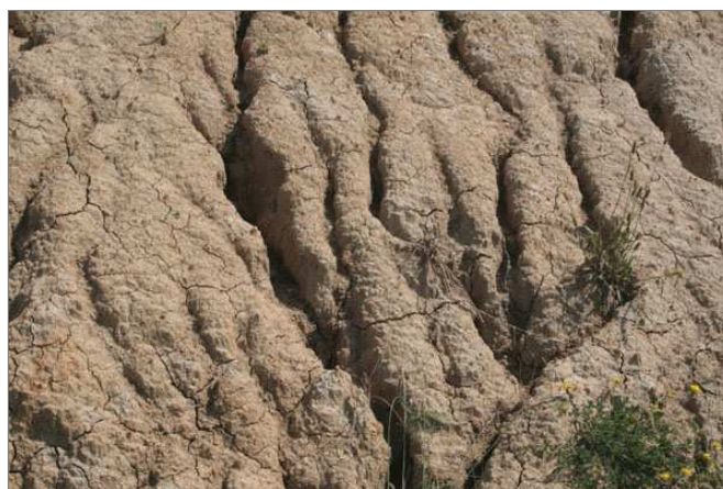
Fig. 2. Flow ditches and rills (Nicolae Lazăr)
