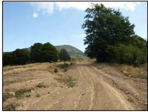
Fig. 2b. Linear erosion processes on forest roads
